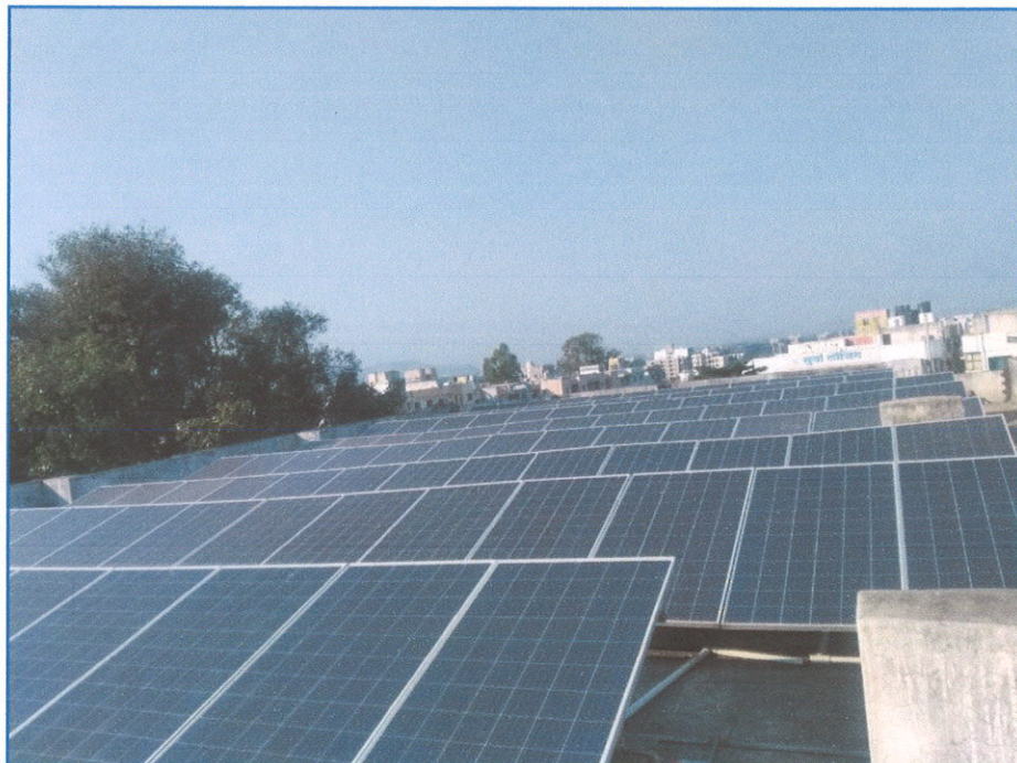
Photographs 8 : Solar System Installed at Institute
